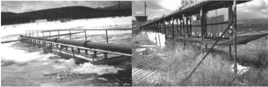
Inca Grid Aeration System in Operation and in Dry Pond
