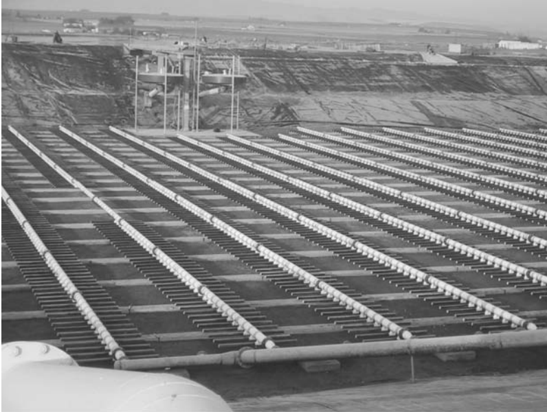
FIGURE 4.34 Ashbrook Lagoon sequencing batch reactor (SBR), Quincy, Washington. (From Burnett, C.H. et al., Ammonia Removal in Large Aerated Lagoons, paper presented at WEFTEC Annual Meeting, Water Environment Federation, New Orleans, LA, October, 2004.)
