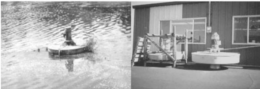
Floating Aerator in Operation and Out of Service
