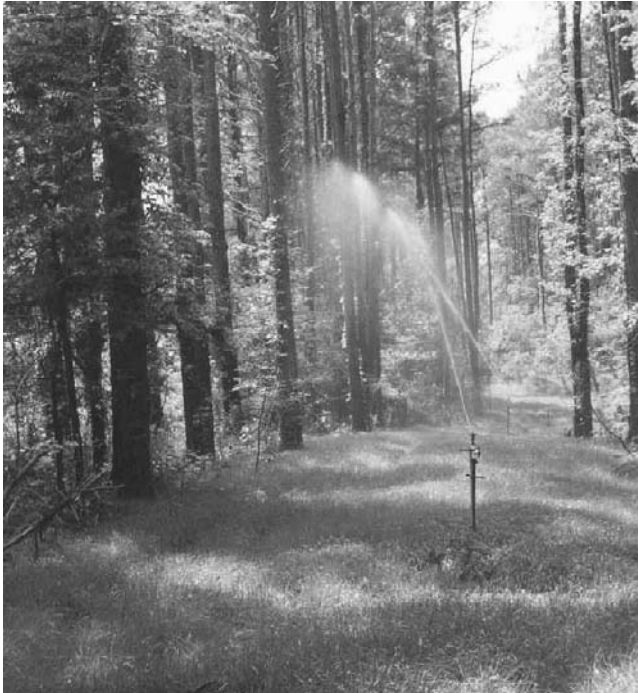
FIGURE 8.1 Typical sprinkler irrigation system at the forested slow rate site at Dalton, Georgia.
