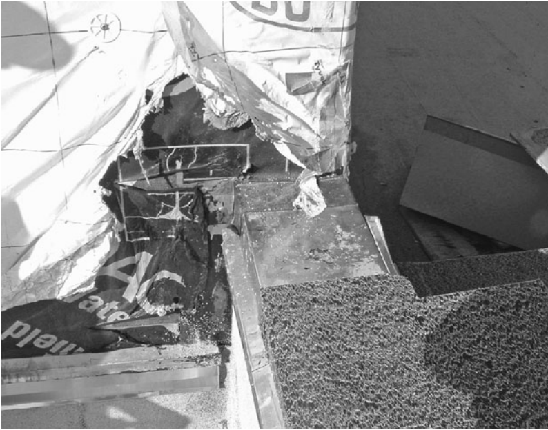
Figure 1-31 Melted wall membrane from torch applied roofing.
