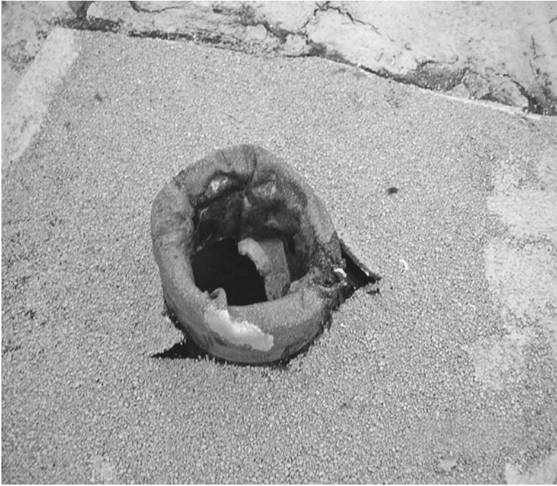
Figure 6-15 Plumbing vent stack, photo.
