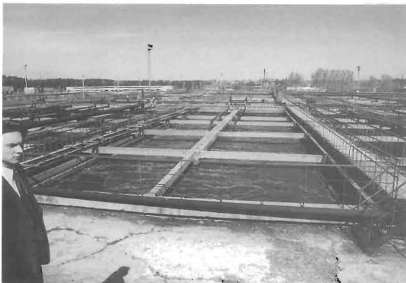
Figure 8. Rectangular settling basins in operation.
