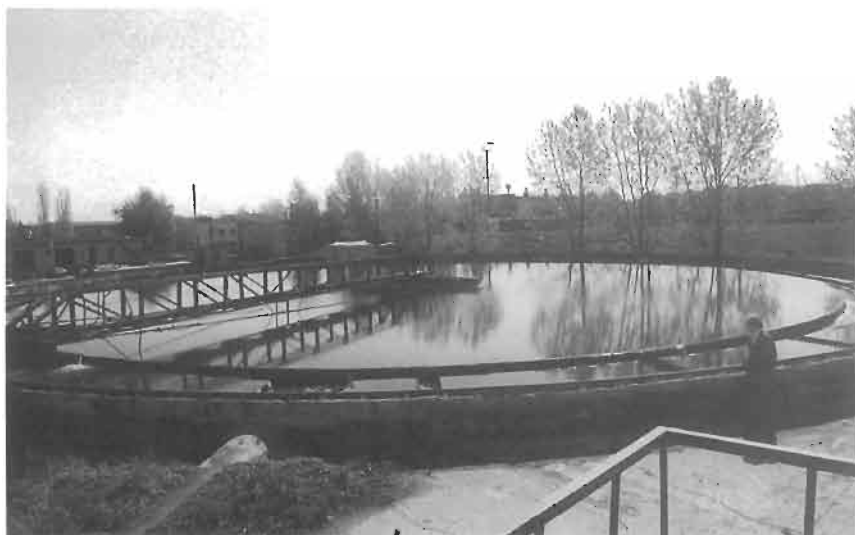
Figure 7. Clarifier used in a wastewater treatment plant.
