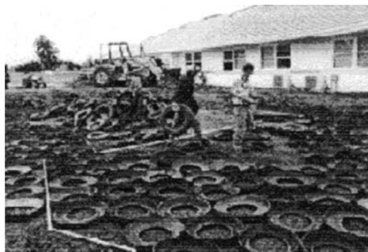
Fig. 8 Rain trap system using split scrap tires to collect and reuse irrigation water in Santa Rosa, California, installed May 1996
