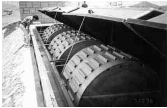
Photo 4.1 Rotating biological contactor.
