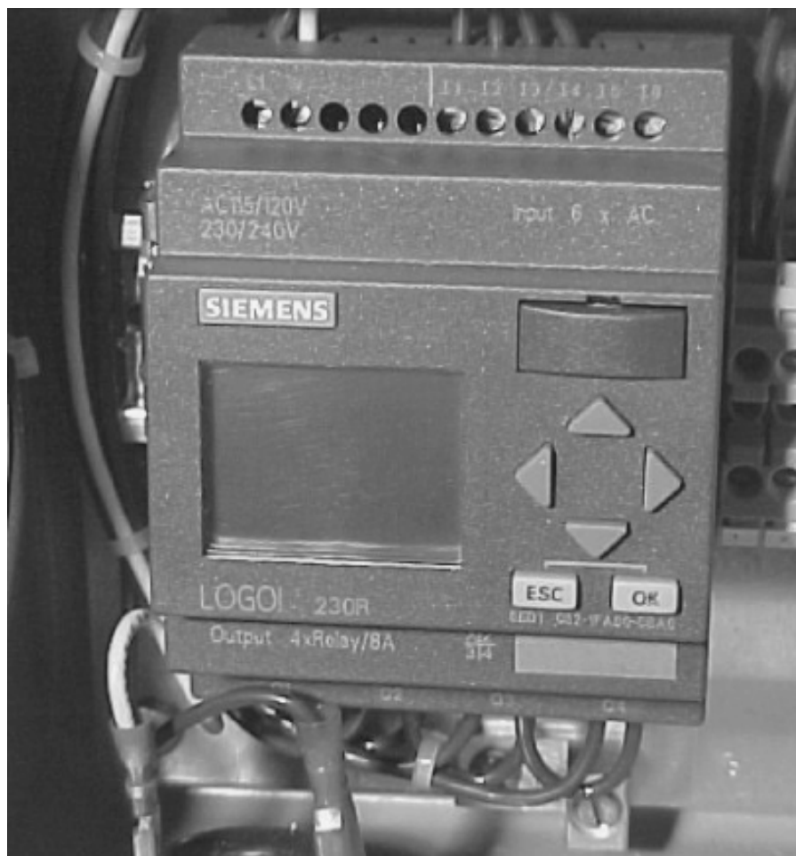
Photo 3.2 Programmable logic controller
