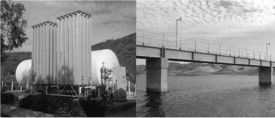
FIGURE 5.22 Lake Bard hypolimnion oxygenation system. (From American Academy of Environmental Engineers, 2005 Project and photo by Kennedy/Jerks Consultants.)
