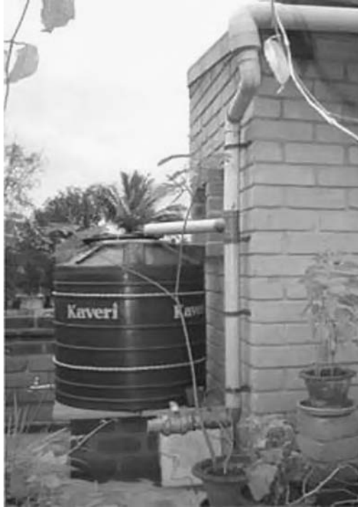
FIGURE 9.12 Storage of rooftop runoff. (From India Together, 2005; photo by S. Vishwanath.)
