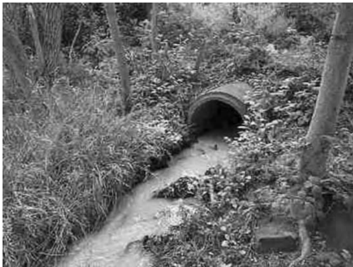
FIGURE 1.5 Stormwater outlet. (From Rogue Valley Council of Governments, 2000.)
