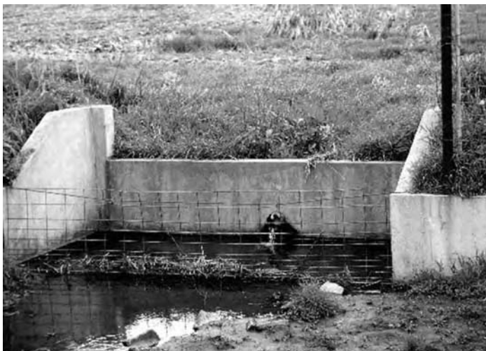
FIGURE 9.42 Drop structure. (From NRCS, 2005e.)
