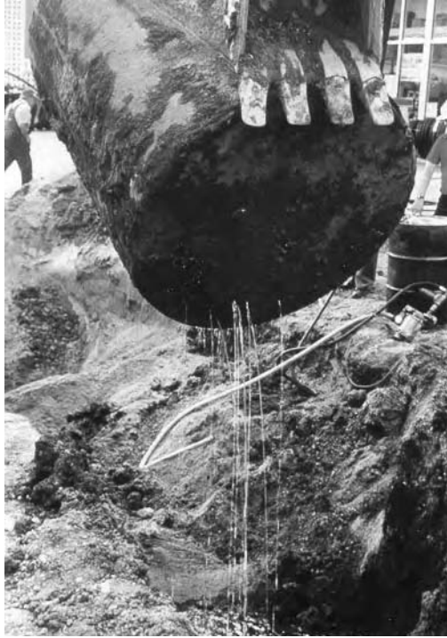
FIGURE 7.3 Leaking underground storage tank. (From USEPA, 2005e.)
