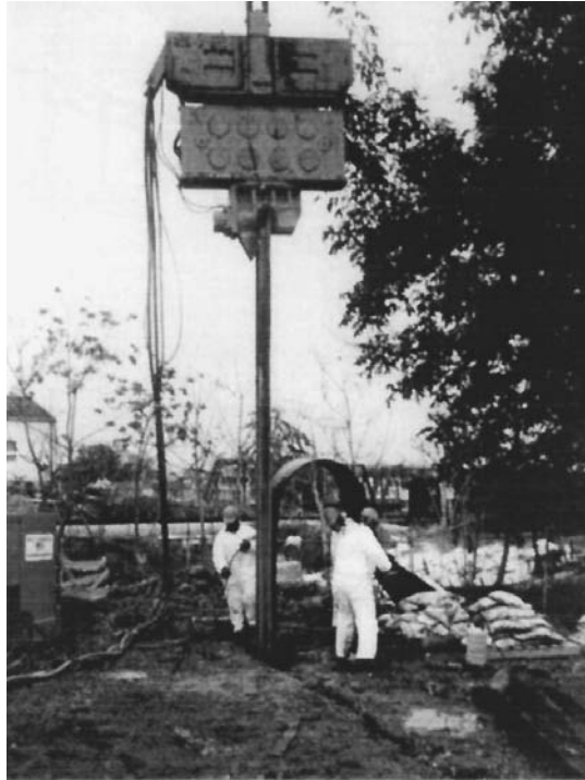
FIGURE 27.20 Installation of HDPE barrier wall utilizing conventional pile driving equipment. (Photo courtesy of Groundwater Control, Inc.)
