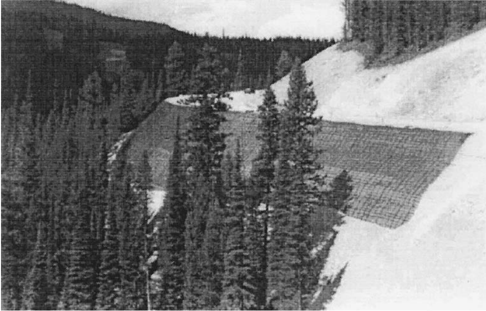
FIGURE 27.16 Erosion control mat placed to help establish the vegetation on the face of a 1H:1V reinforced soil slope.
