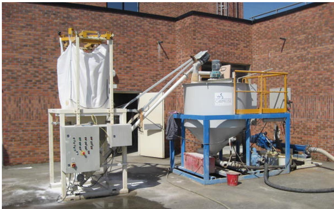
Fig. 7: Pilot unit for CODECAL ® process testing
