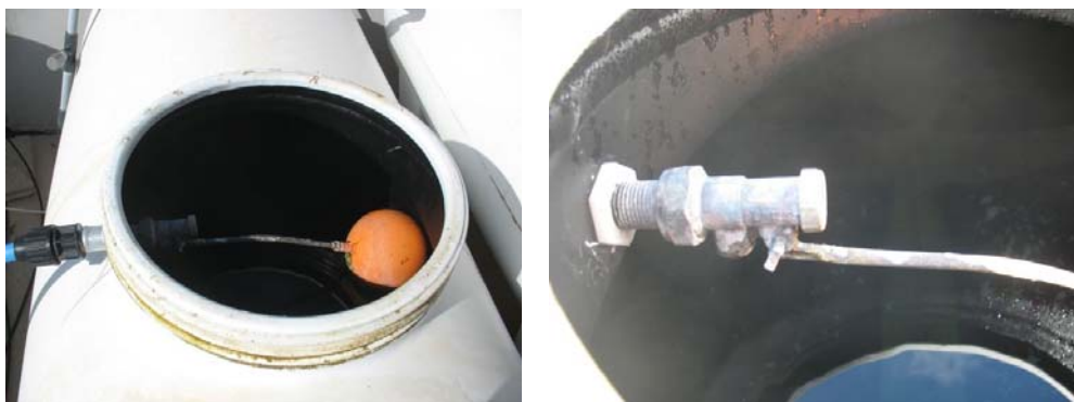
Figure 4. Polypropylene Roof Tank
