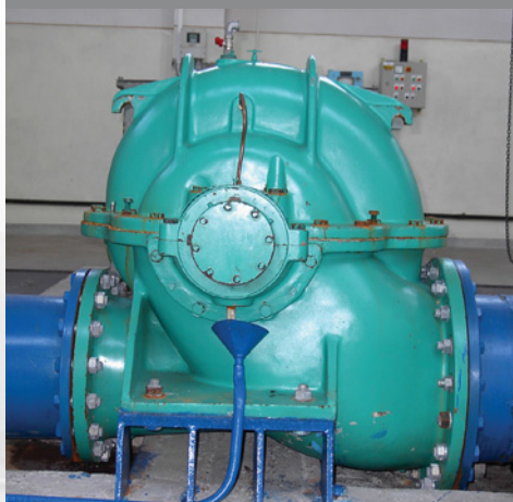
Stații de pompare Pumping Stations Pumpwerke
