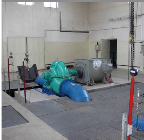
Stații de pompare Pumping Stations Pumpwerke
